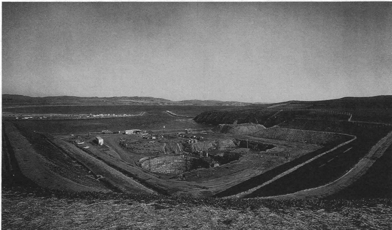
5. Excavation for proposed reactor at Bodega Head, California. The harbor is immediately in front of the construction area; the mainland is in the background. (AEC Docket 50-205)
