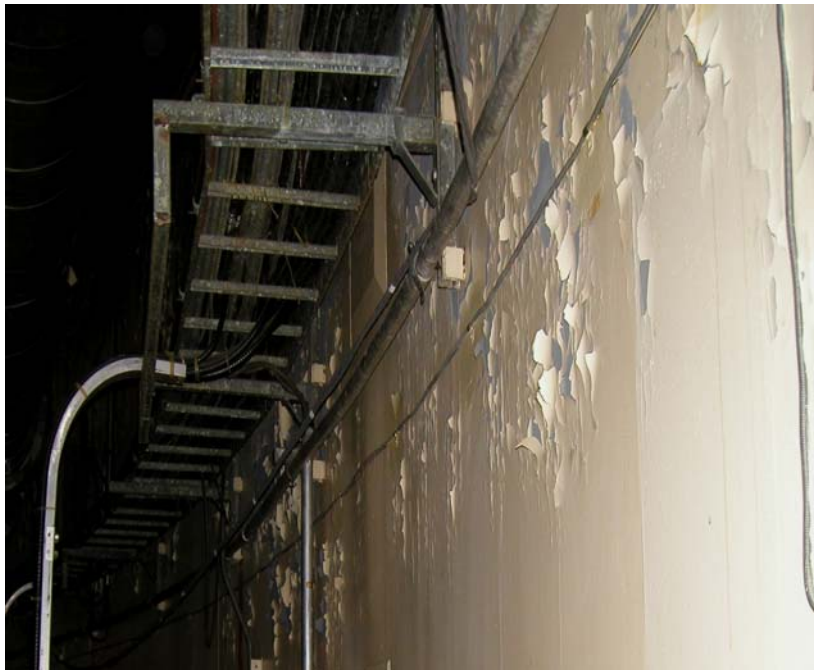
Figure 4 Example of Coatings Degradation at Oconee
